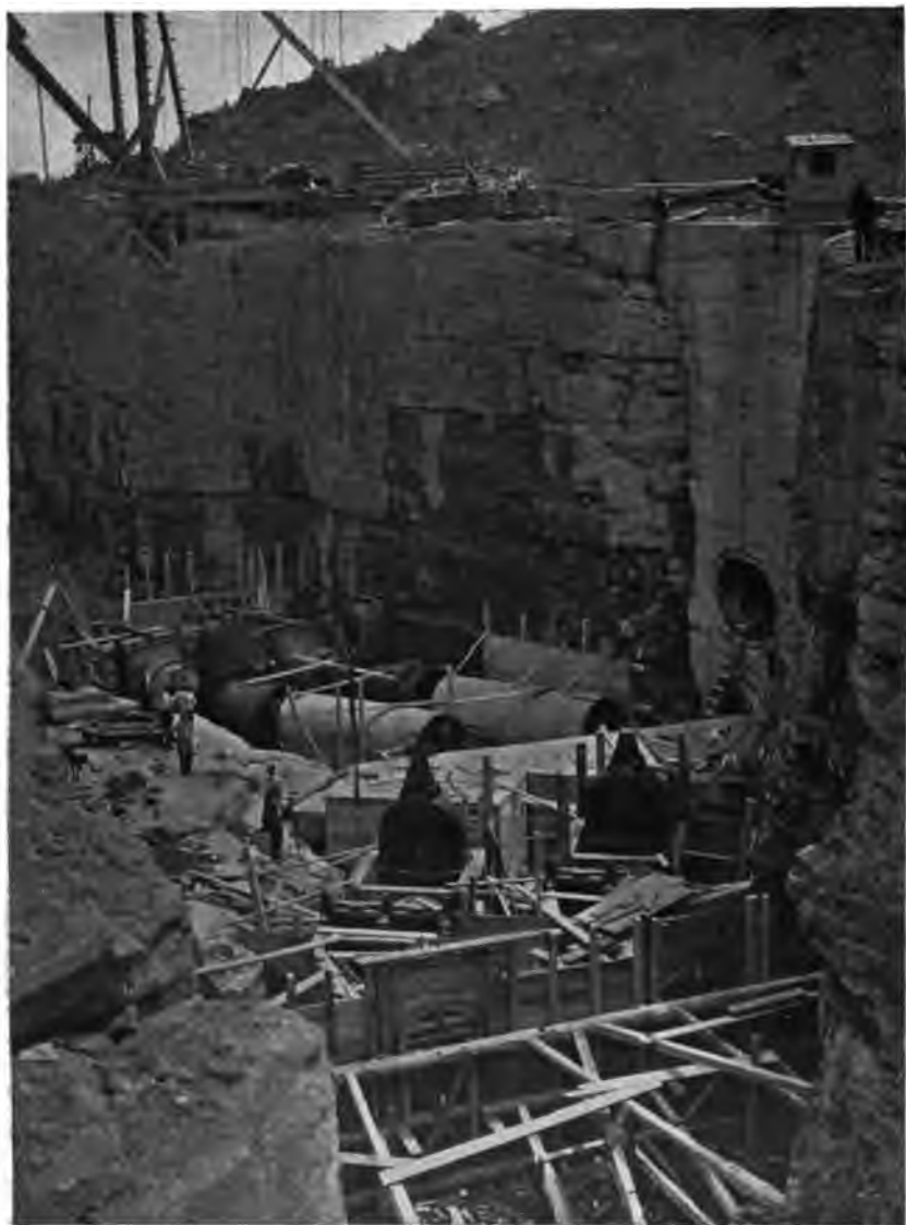
PLATE 57. —View of Upper Gate Chamber, Upper and Lower Special Aqueducts, for Draining Water from Reservoir under Dividing Weir Dike at Right, 60-inch Gate Valve being Placed. Contract 3.
